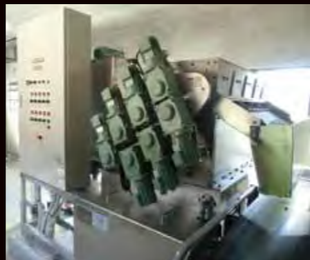
Excess Sludge at Noodle Production Plant (JD-1000)
